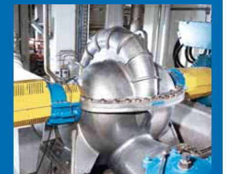
▲ Headbox pump with efficiency of 91% and very low pulsation (installed on PM1 at Myllykoski Continental GmbH in Plattling, Germany).
