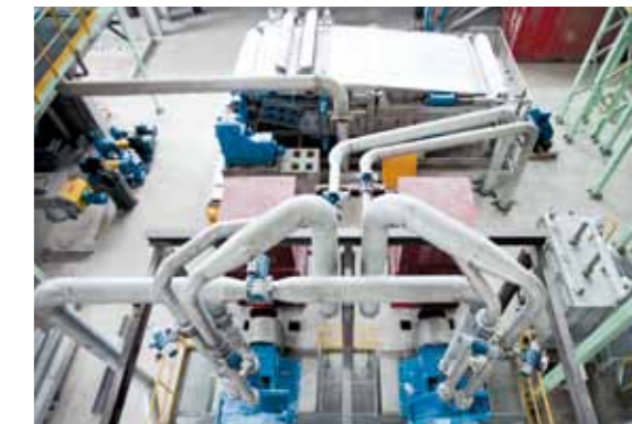
ANDRITZ LC refining inside the new BCTMP building. ▼
