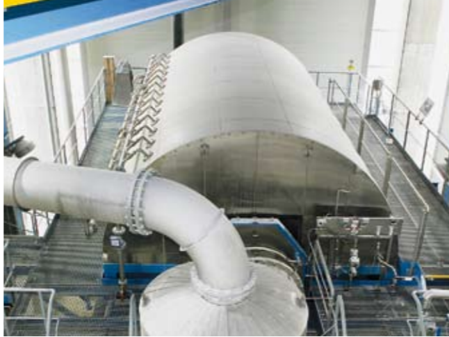
▲ The two-stage washing capability of the LMD-Filter™ from Andritz is meeting the mill's requirements for lime mud dryness and low emissions perfectly, according to Michael Bauer, Assistant Production Manager.
