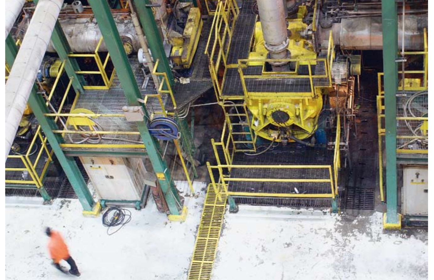
▲ One of four Andritz Twin™ 50 refiners in the secondary position at Augusta Newsprint. The TMP plant produces 1100 t/d for the mill's two newsprint machines.
