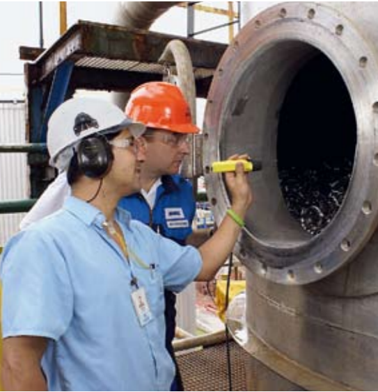
Looking inside the condensing scrubber vessel on the CBC boiler are Isaias Shimura, Recovery Process Engineer for Suzano (left) and João Guilherme Heinz Cruz, Service Engineer for Andritz. ▲
