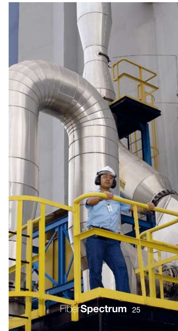
The Andritz DTVG technology installed at Suzano conditions the gases in the smelt dissolving tanks so they can be burned in the recovery boilers. TRS emissions from the tanks are eliminated. ▼
