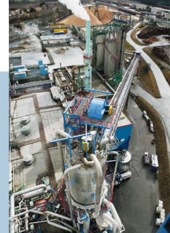
▲ The fiberline at Pöls has been upgraded several times over its life and currently produces about 1150 adt/d. Andritz supplied a Diamondback® chip silo to upgrade the feed to the digester.
